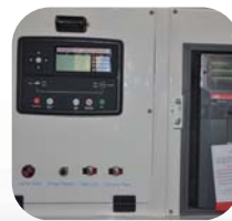
Control Panel & MCB
